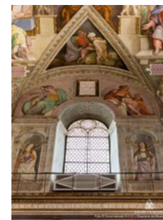
Air-to-air heat pump installation in Sistine Chapel, Rome
